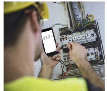
Electric Power Inspection
